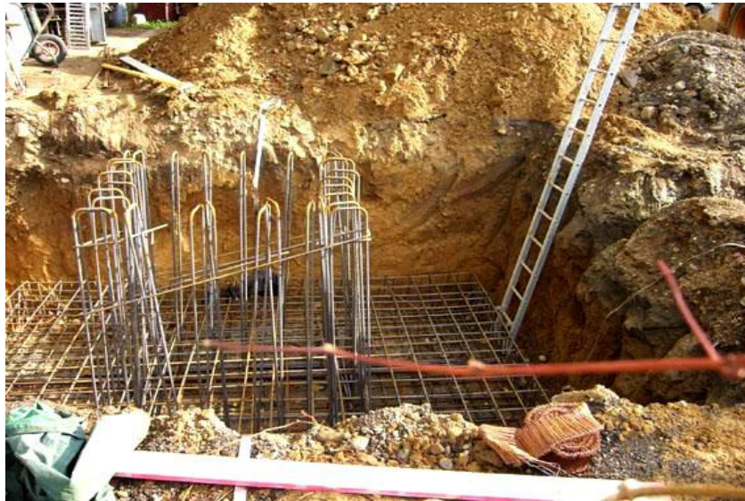
Reinforcement for the foundations of the concrete pylon used to disguise the Bouygues Telecom antennas (Tassin la Demi-Lune)
