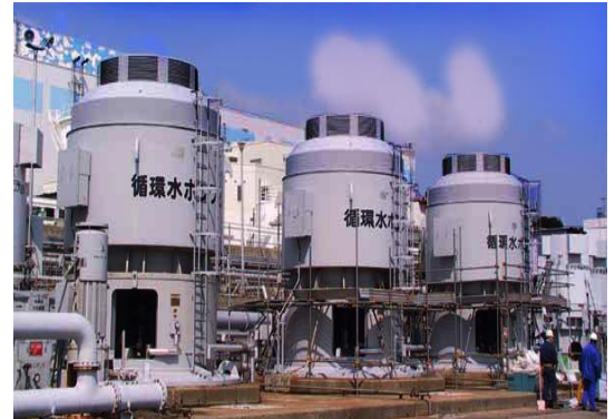
Giant vertical pumps water cooling reactor at the Fukushima Daiichi nuclear power plant. (Photo TEPCO)
