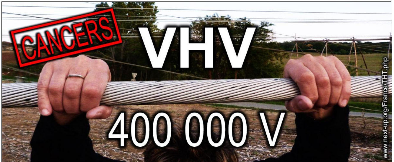
France : Aerial cable line VHV 400 000 V
