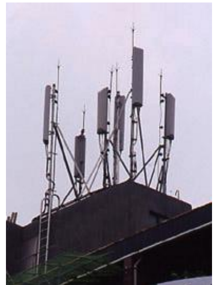
Taiwan : Base stations and microwave receivers installed on building roofs have aroused concern about the potential effect of electromagnetic waves on area residents
